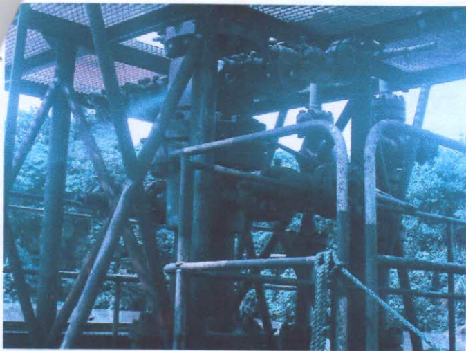
Figure 1: TUNU WELLHEAD 4 VIEWED FROM RIGHT POSITION.
